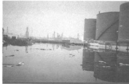
Figure 1. In 1990, a tank foundation collapse at an Amerada Hess facility in Perth Amboy, New Jersey, USA led to tank failure that created a 6 million gal. lake of oil around the damaged unit.
