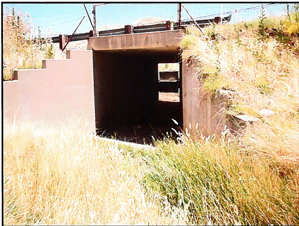
Box culvert under Kirker Pass Road at the north tip of the wetland swale, looking northeast; 06/28/10.
