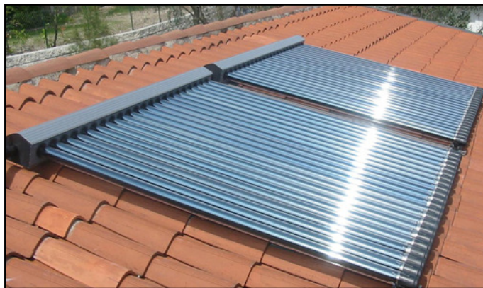
Solar Hot Water System
