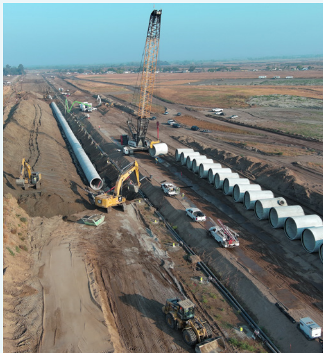
Contra Costa Water District recently replaced the beginning section of the Contra Costa Canal with a 10-foot diameter pipeline. This project improves public safety, water supply resiliency, and water quality.
