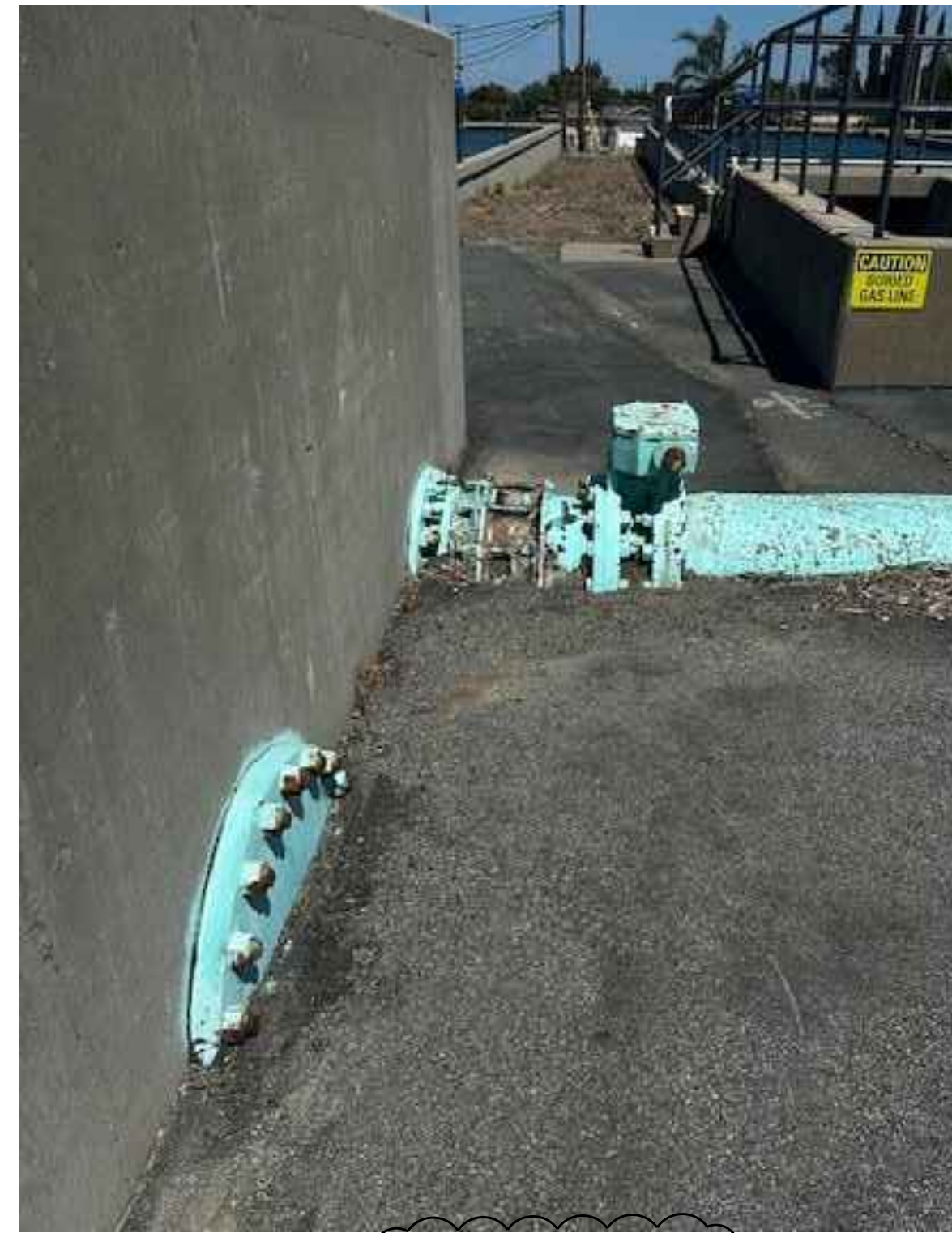
PICTURE 1 EXISTING 24" BFV (VIEW FROM EAST)
