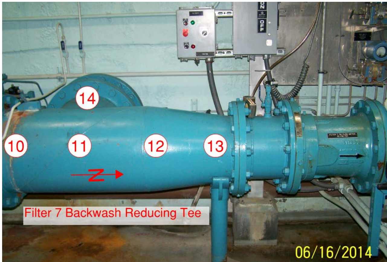
Figure 2-4. Filter 7 Backwash Reducing Tee Measurement Locations
