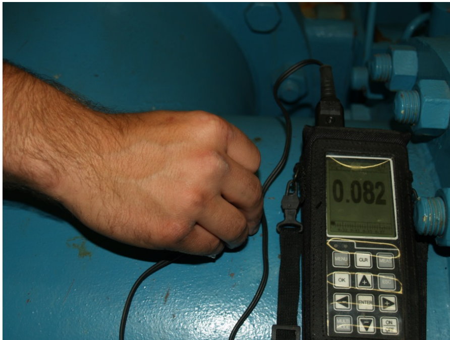
Figure 2-8A. Ultrasonic Thickness Tester at Thin Spot at Filter 8 Tee (Location with a measured thickness of less the 0.10 inches)
