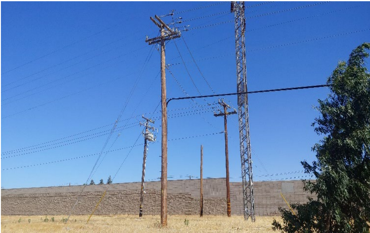
Utility Poles on the project site
