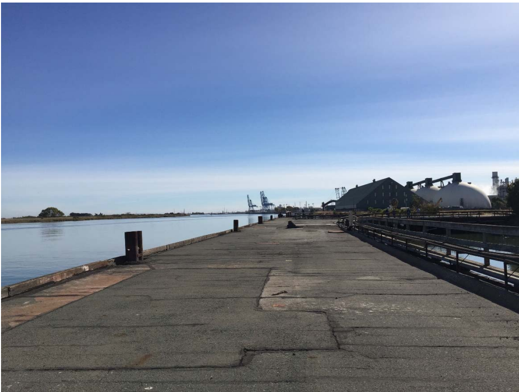
Terminal platform view
